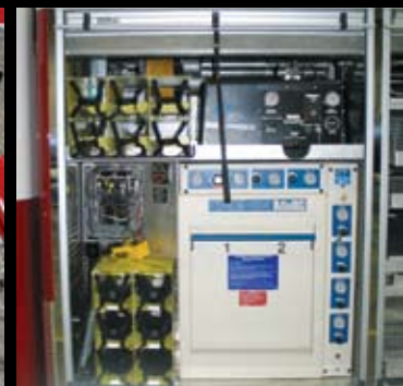
Breathing air fill station and storage
